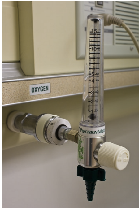
Fig. 4.3 An oxygen flowmeter inserted into the wall outlet
